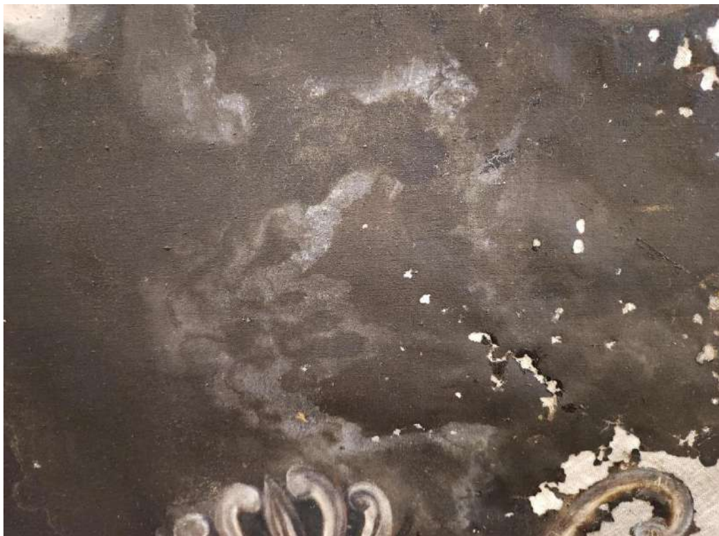
Details of the crystallized salts present on the surface.
