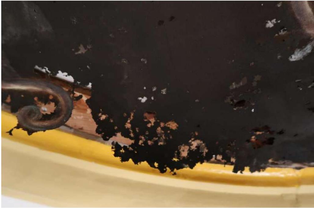
Detail of the fabric before restoration. The loss of original support in the affected area caused it to hang down with no contact with the frame.
